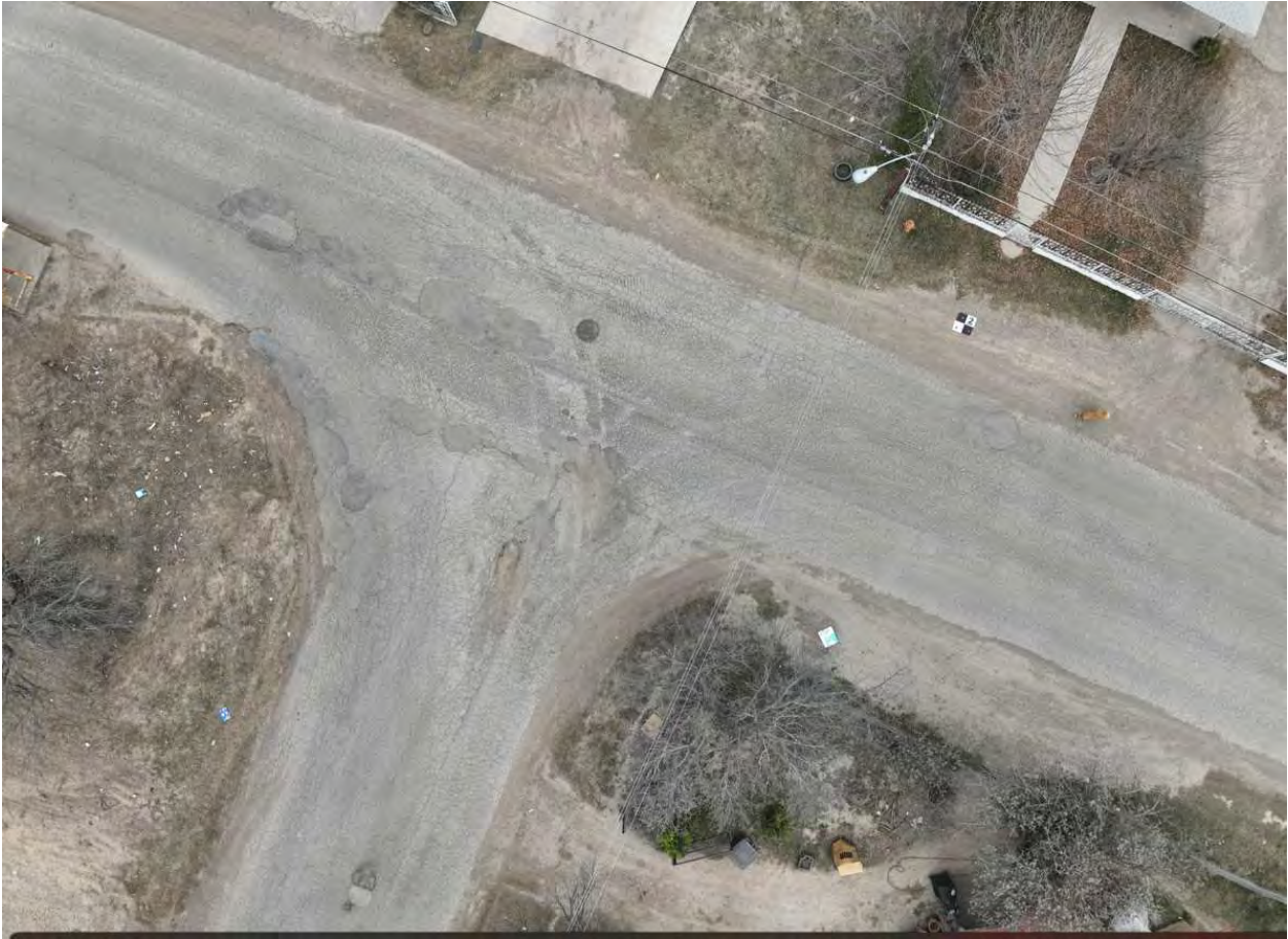
Figure 5. View from the south of La Herradura road, the no curb and no sidewalks within the vicinity of the property.
