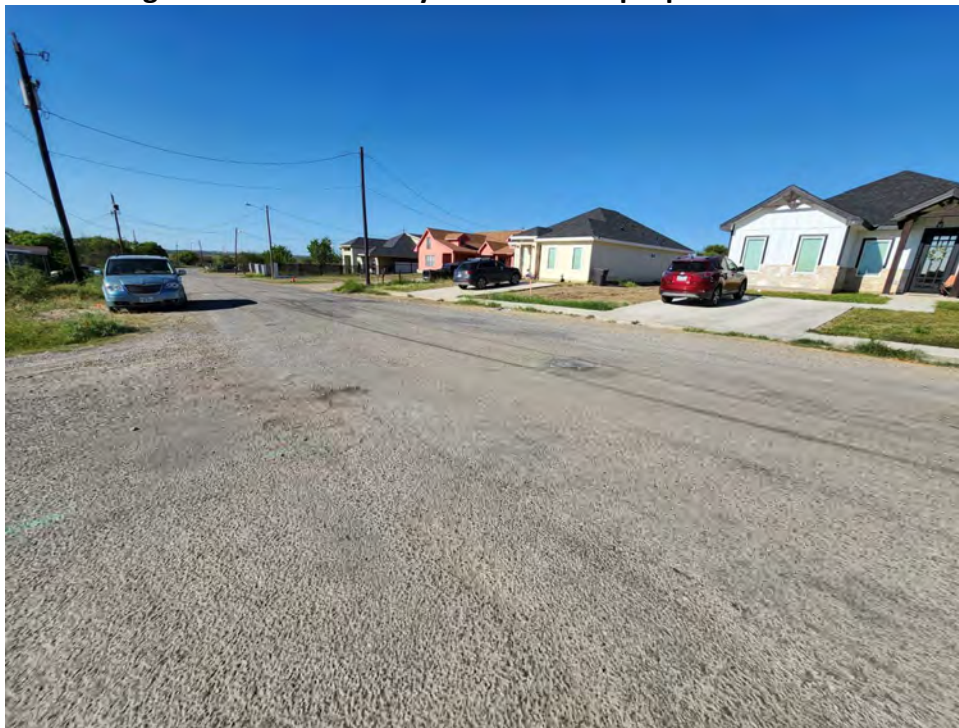
Figure 10. Nearest intersection, showing no curb and gutter in the vicinity.
