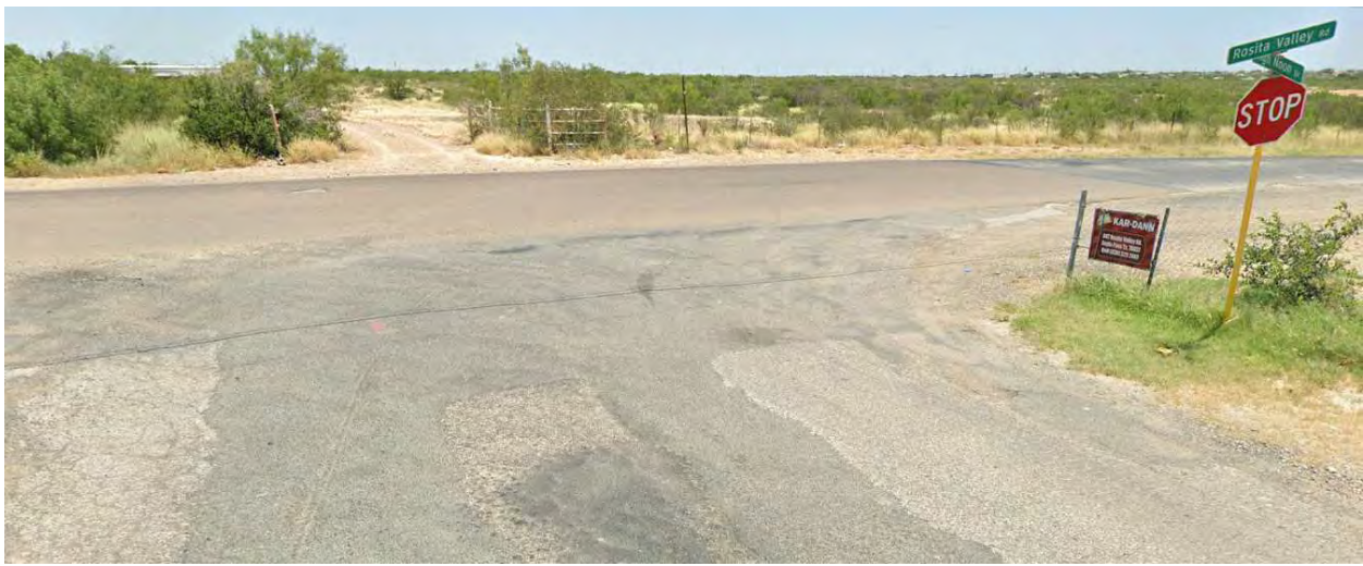
Figure 9. Nearest intersection, showing no curb and gutter in the vicinity.
