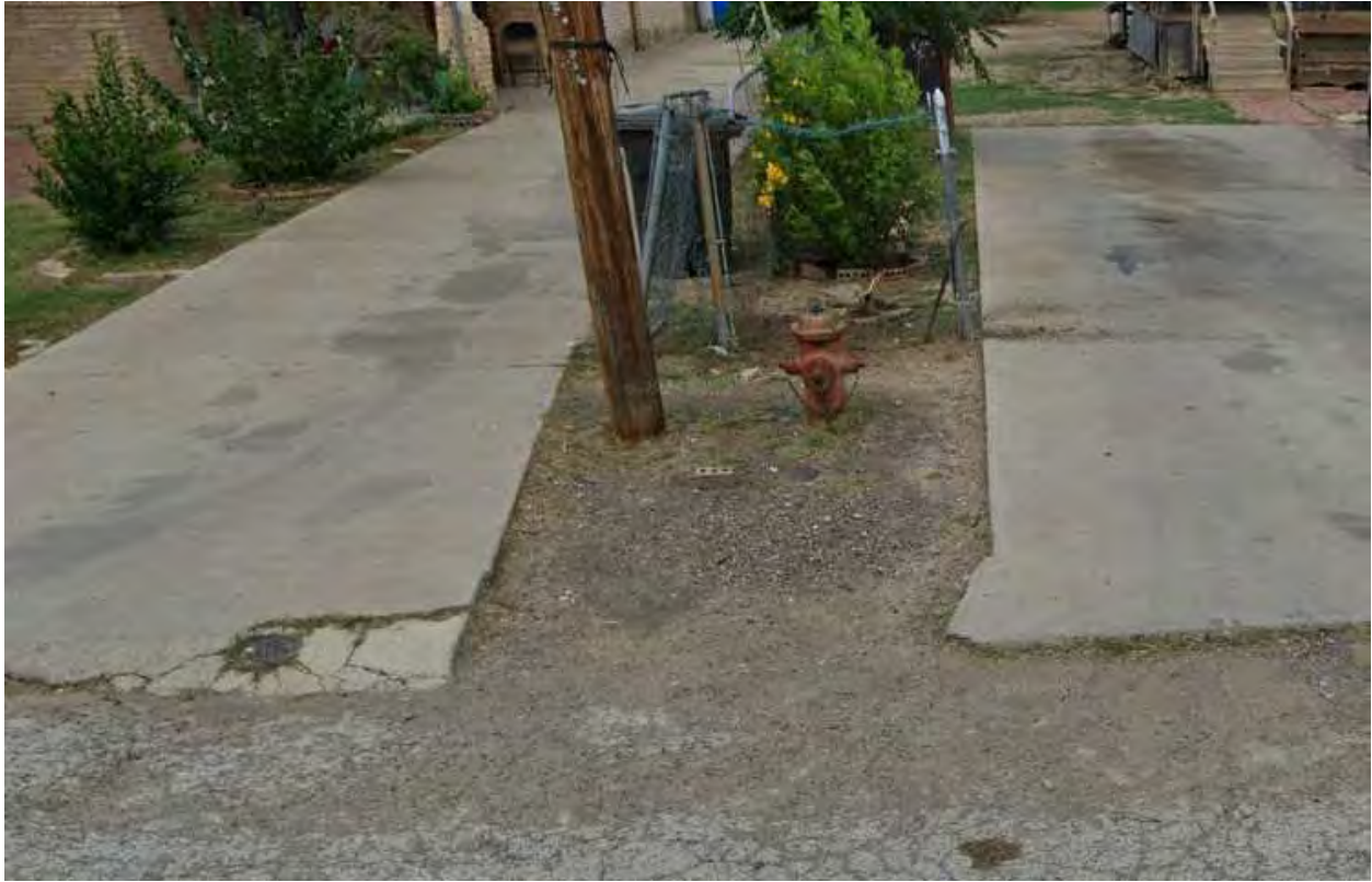
Figure 9. Fire Hydrant located across La Herradura road, on the northeast corner of the property
