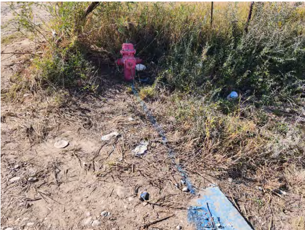
Figure 9. Fire Hydrant located on the east boundary of Lot 1
