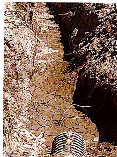
Detention Pond Outlet
